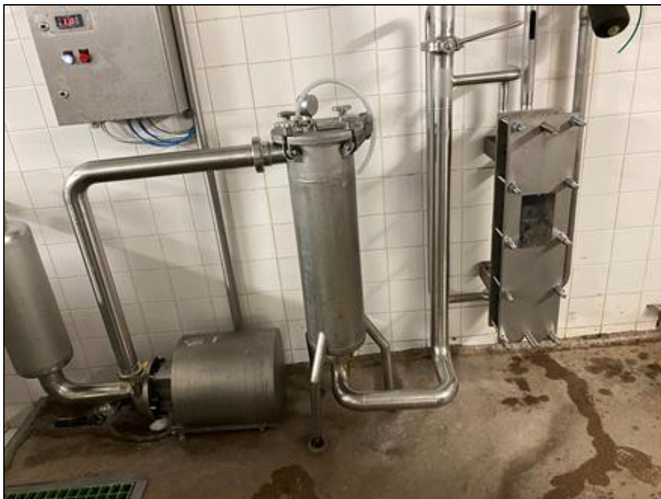
Brine cooler and filter system
